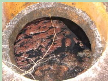
The high level of tank contents indicate that the tank has backed up.
