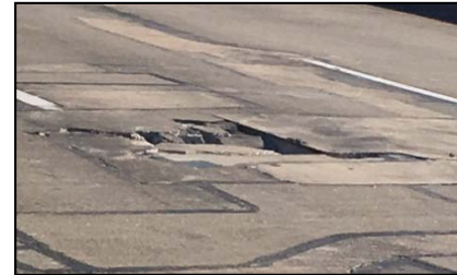
Hole Through Bridge
