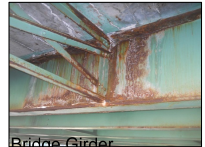
Bridge Girder Corrosion
